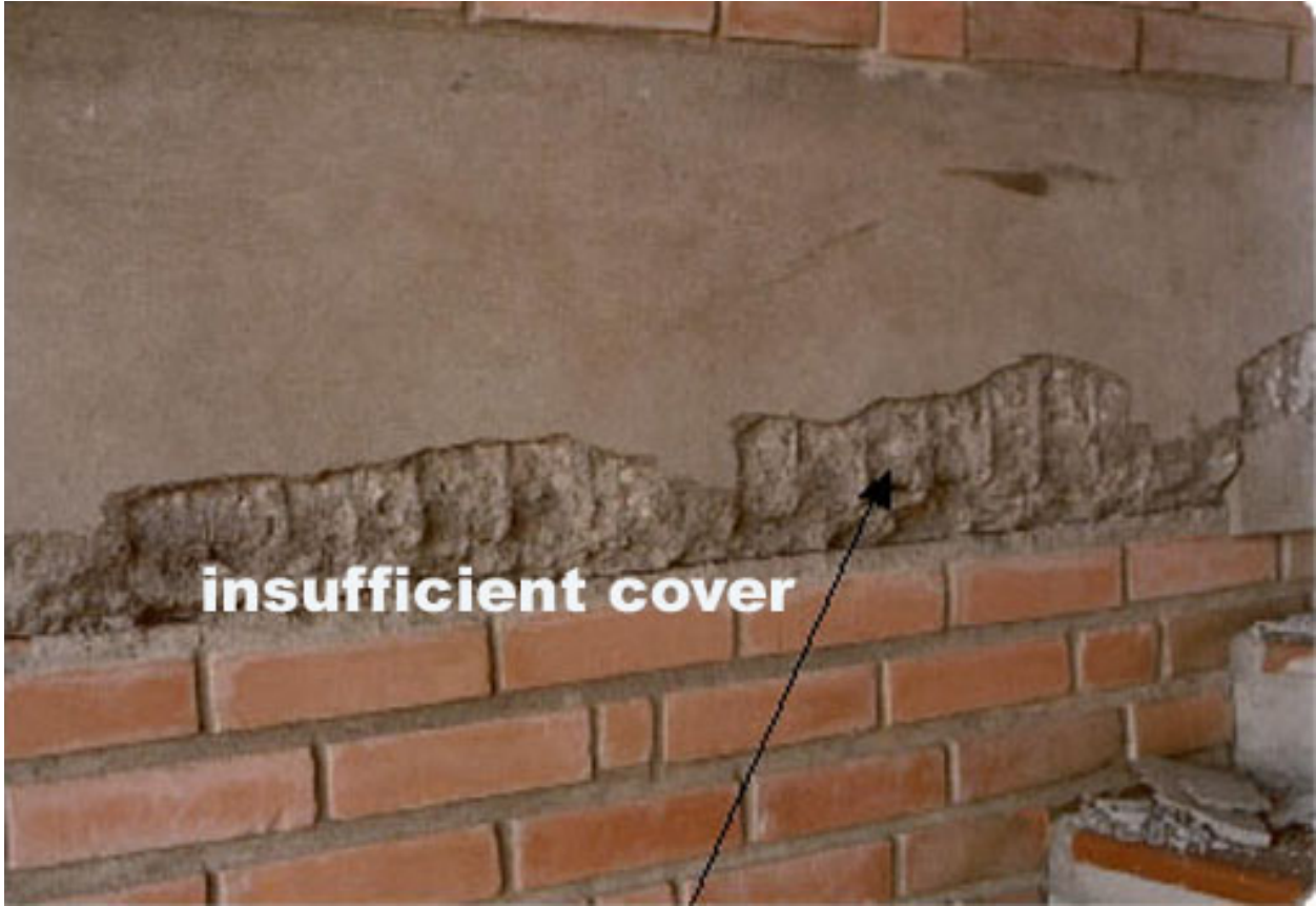
FIGURE 6K: Earthquake Damage: Inadequate Concrete Cover
