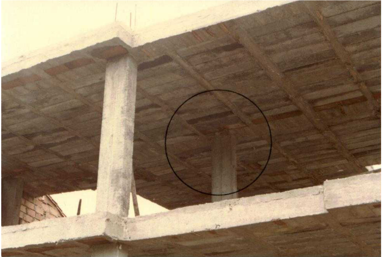
FIGURE 5B: Poor Construction Practice: Beams constructed in one direction only
