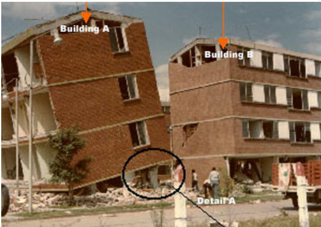
FIGURE 6E: Collapsed building; Detail A shows too widely spaced stirrups
