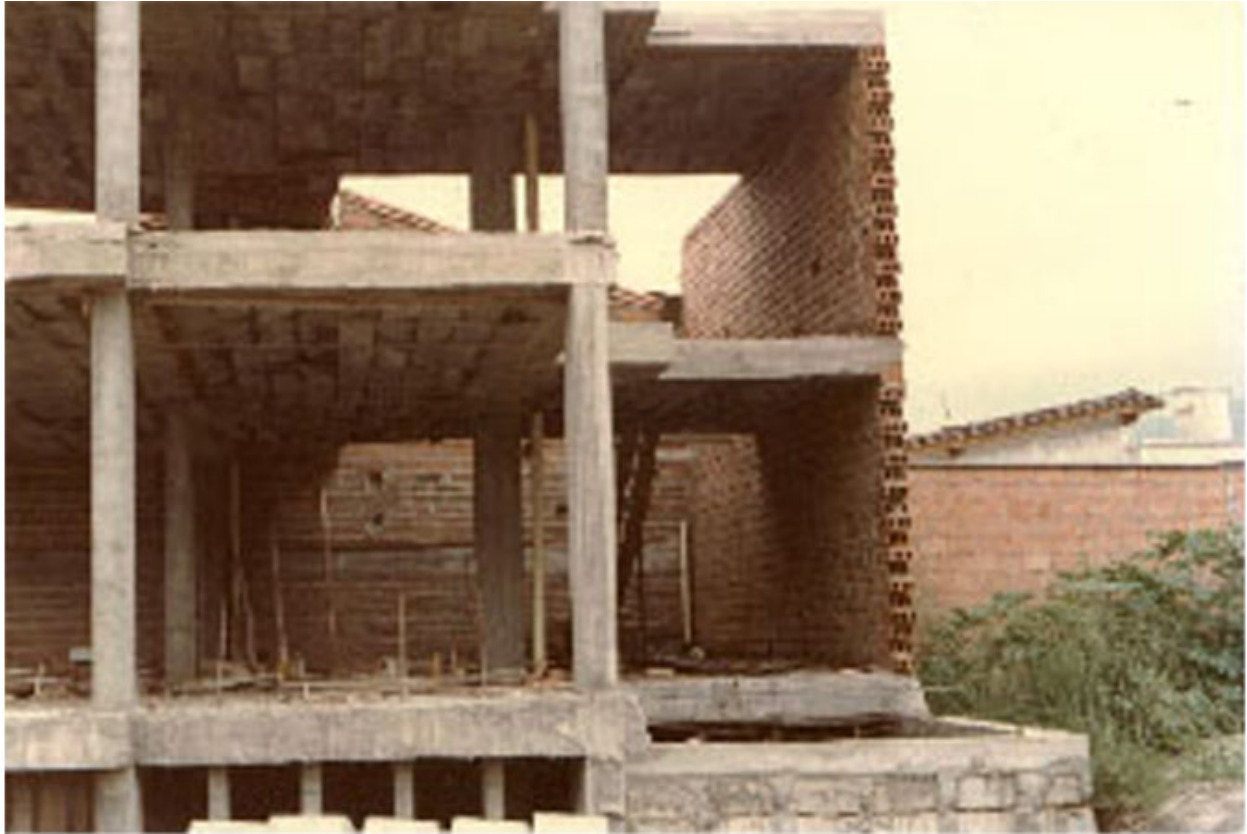
FIGURE 5E: Poor Design: Combination of Concrete Frames and Unreinforced Masonry Walls or Pilasters
