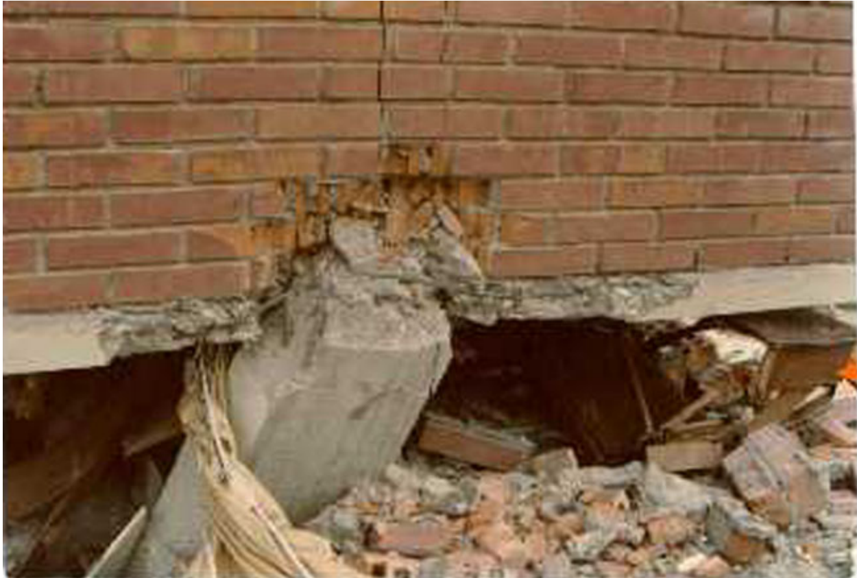
FIGURE 6D: Earthquake Damage: Inadequate longitudinal and transverse reinforcement (Note the collapsed first story.)
