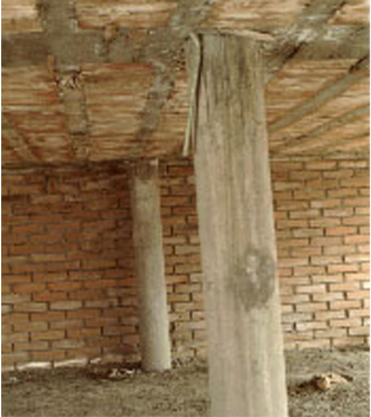
FIGURE 5A: Poor Construction Practice: Beams constructed in one direction only
