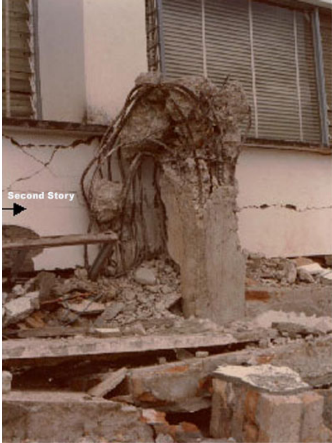
FIGURE 6G: Collapsed 3-story building. (Note the total lateral drift between the 2nd and 3rd floor.)
