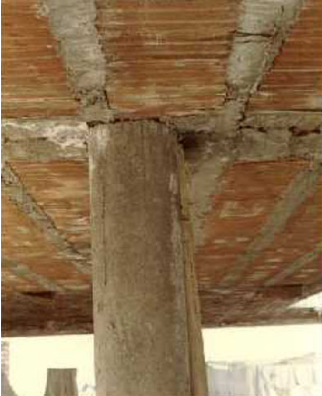
FIGURE 5I: Poor Construction Practice: Drains running across the girders. Stirrups are removed to allow for the pipeline passage.
