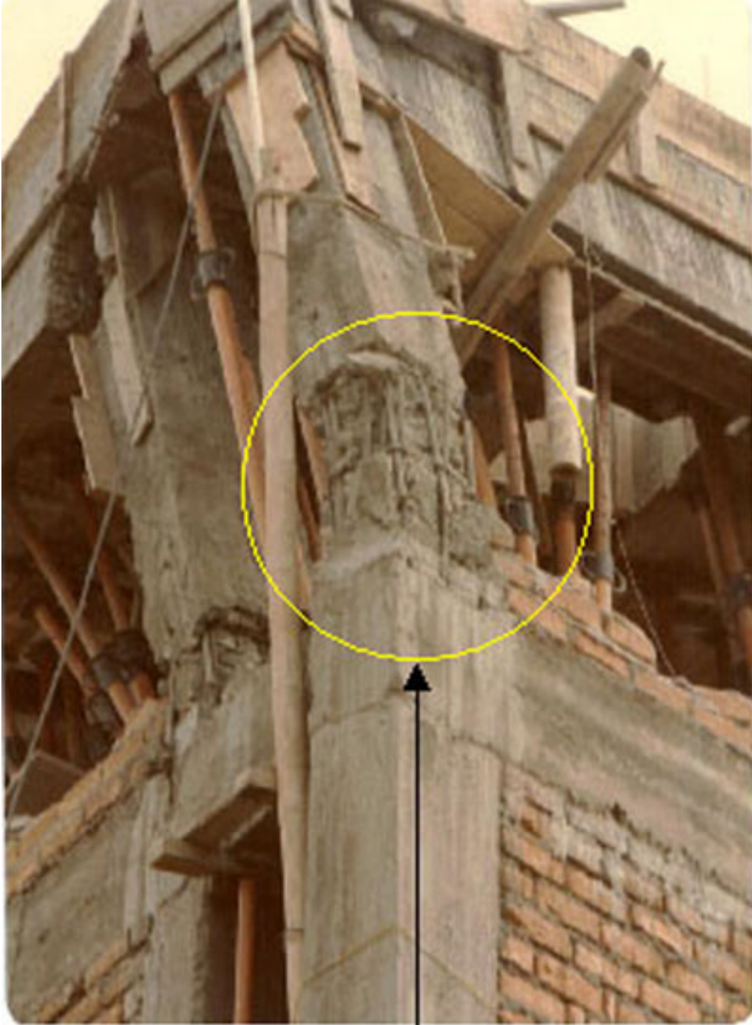
FIGURE 6J: Earthquake Damage: Inadequate Column Splices
