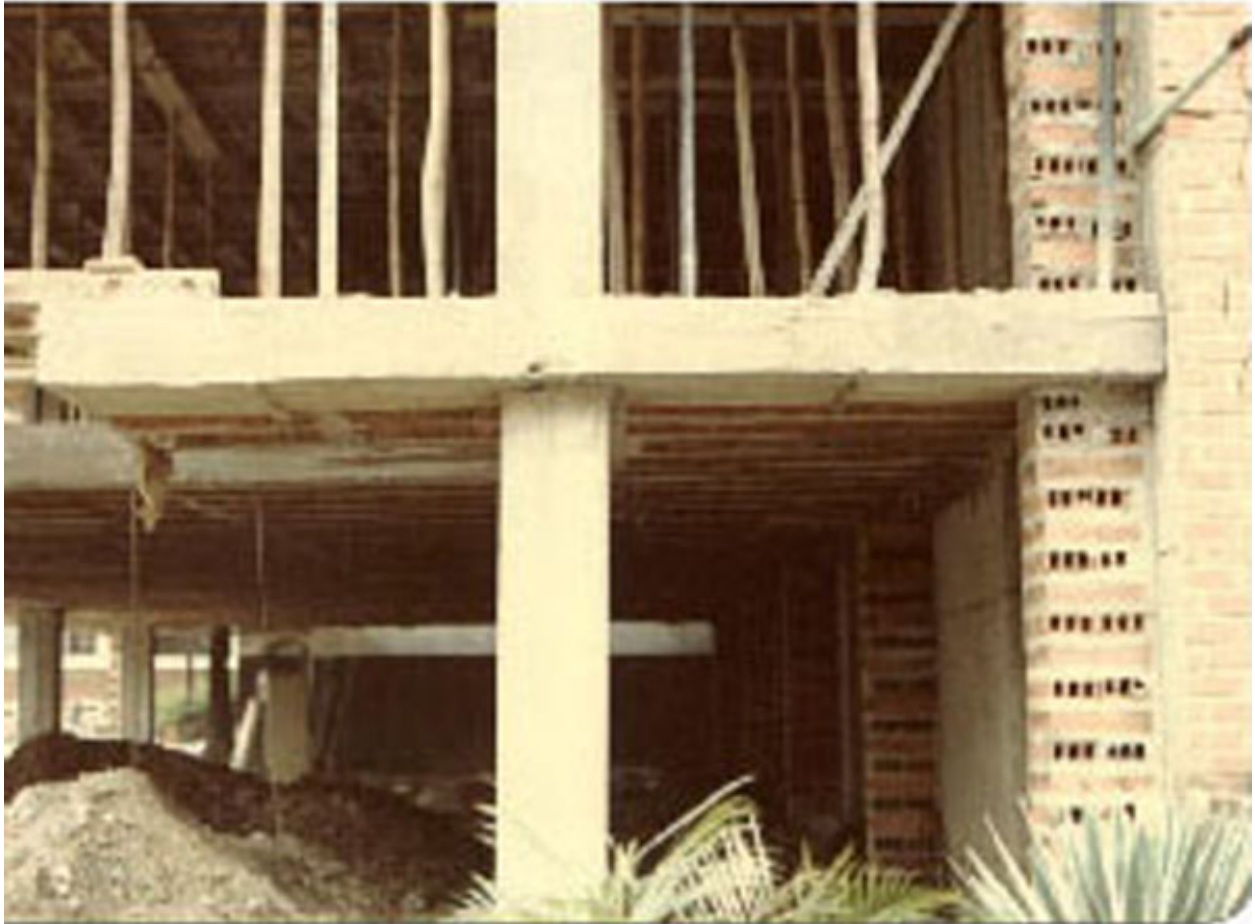
FIGURE 5D: Poor Design: Combination of Concrete Frames and Unreinforced Masonry Walls or Pilasters
