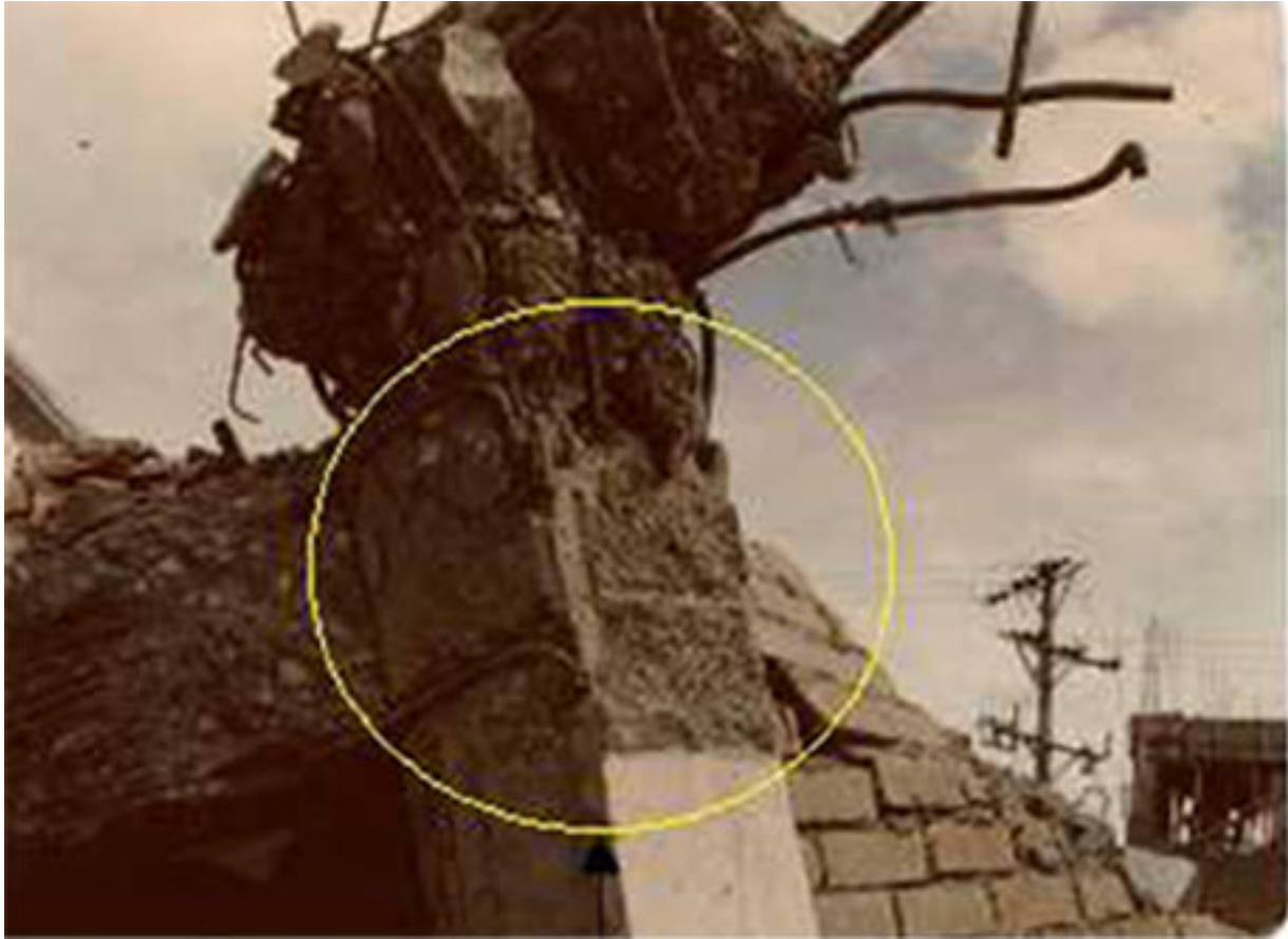
FIGURE 6C: Earthquake Damage: Anchorage of beam reinforcement in the column cover area (It would be correct to anchor the reinforcement inside the joint.) Detail B
