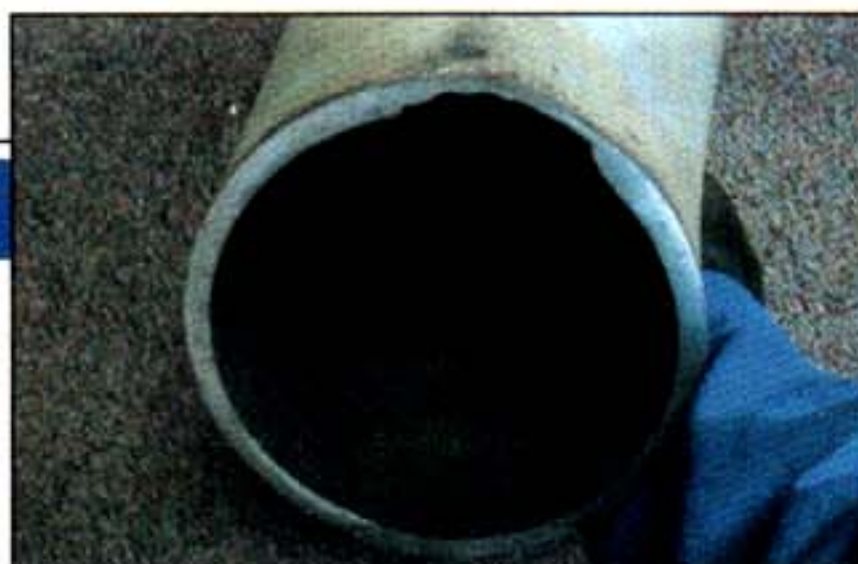
FIGURE 2. The thinner wall at the top of this pipe is characteristic of pipes in stratified-flow service, because vapor and acidic condensation contacting the top can accelerate the corrosion there
