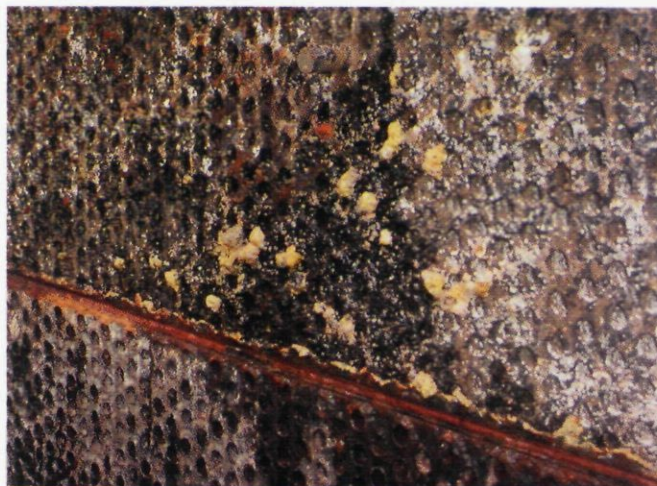
FIG. 1 Inspection of the propylene exchanger shows deposits on the tube sheet after service.
