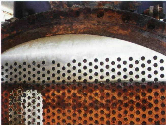
FIG. 6 View of the finished in situ machined to the tube sheet surface.
